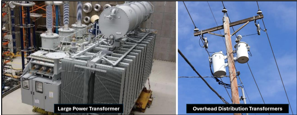
Figure 3: Large Power and Distribution Transformers 10
