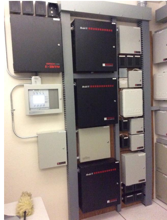
Photo: PACS equipment room. Courtesy of AOUSC.
