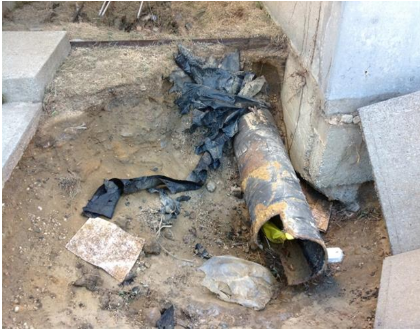
Abandoned Pipe – conduit to flooding of galleries
