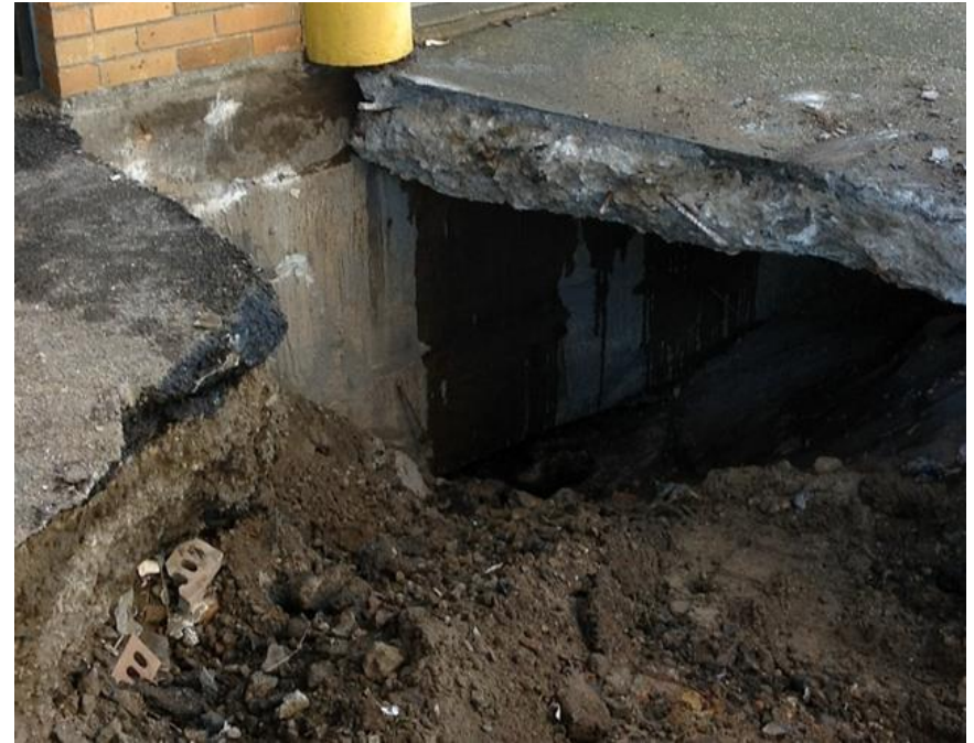
Subsidence at Sludge Storage Bldg
